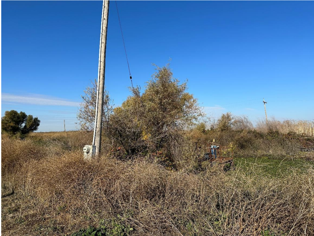
Photo No. 13 Water supply pump in irrigation canal in northern portion of the site
