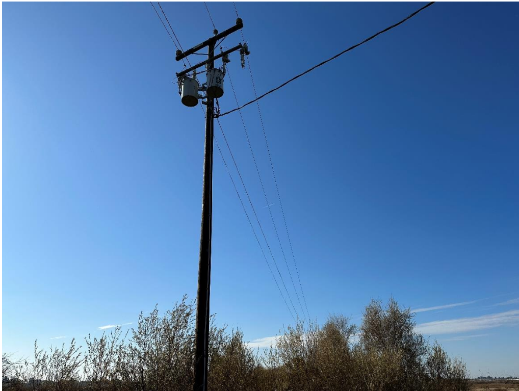
Photo No. 14 Pole-mounted transformer adjacent to water supply pump
