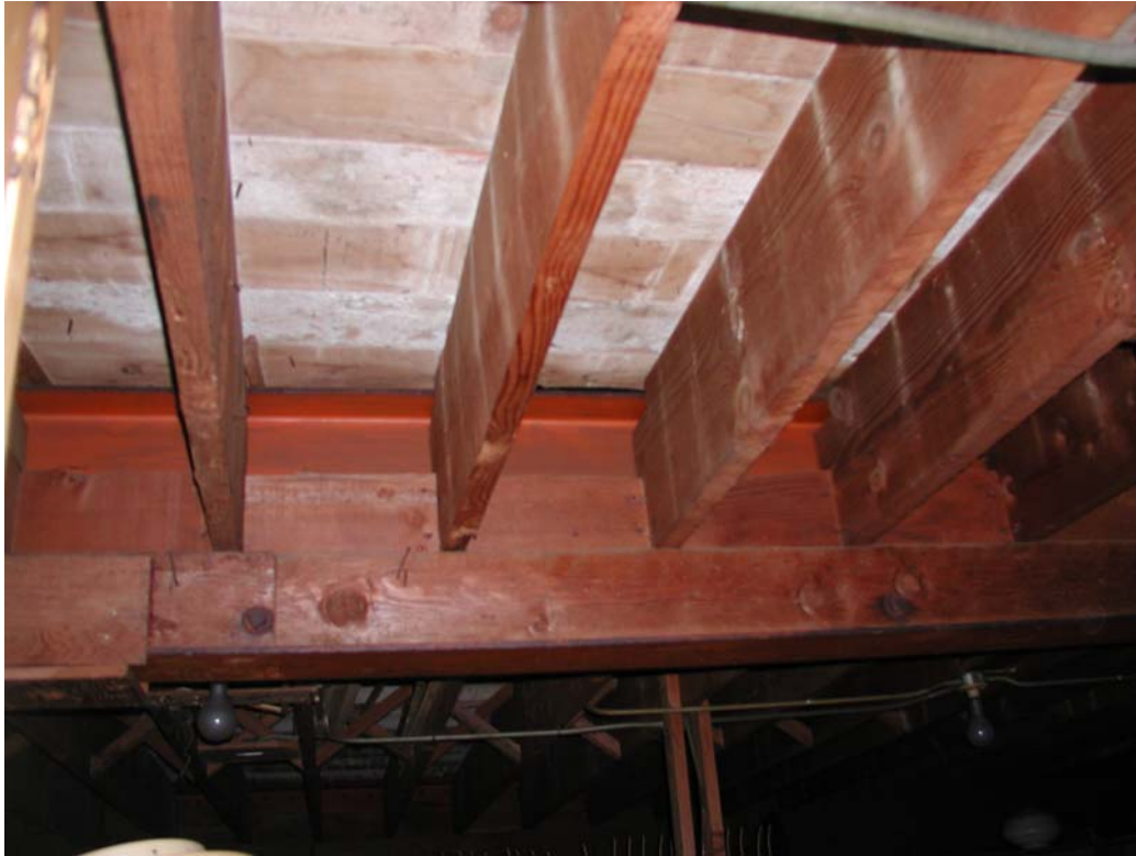
Typical floor framing supported on steel beam and straight sheathing above joists
