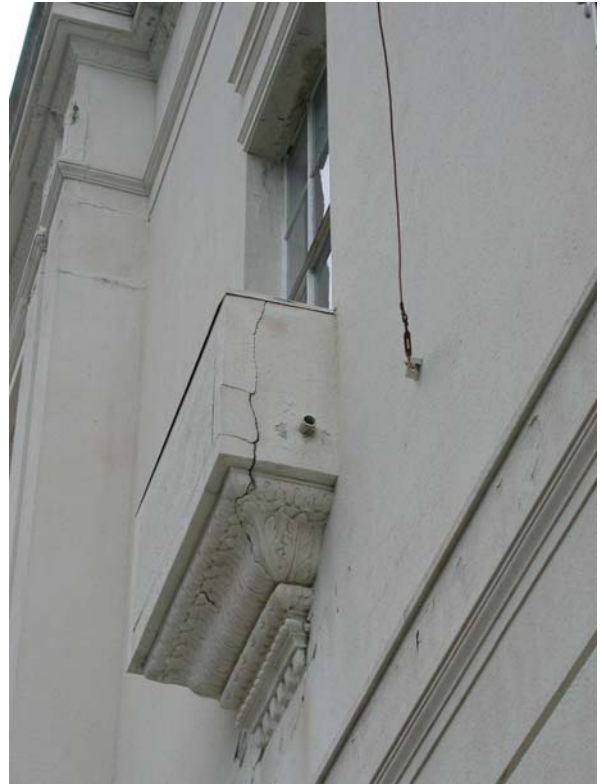
Cracking at Ornamentation
