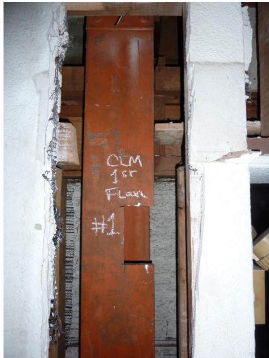
Column with coupon cut from flange (Repair required)
