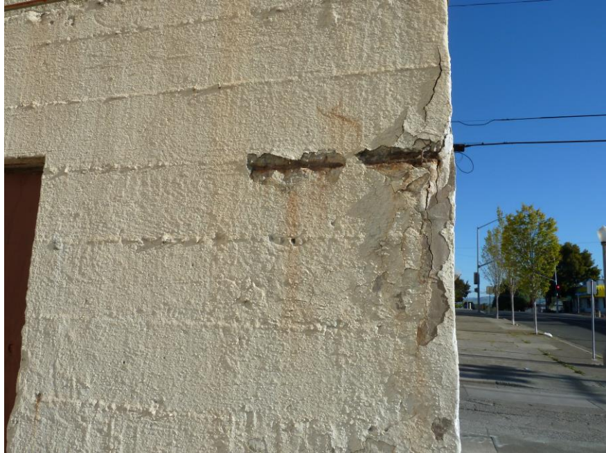
Exposed reinforcing on north façade of east stair tower
