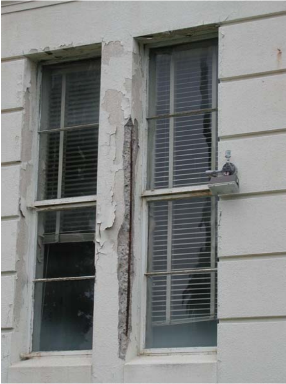
Concrete Spalling at Façade
