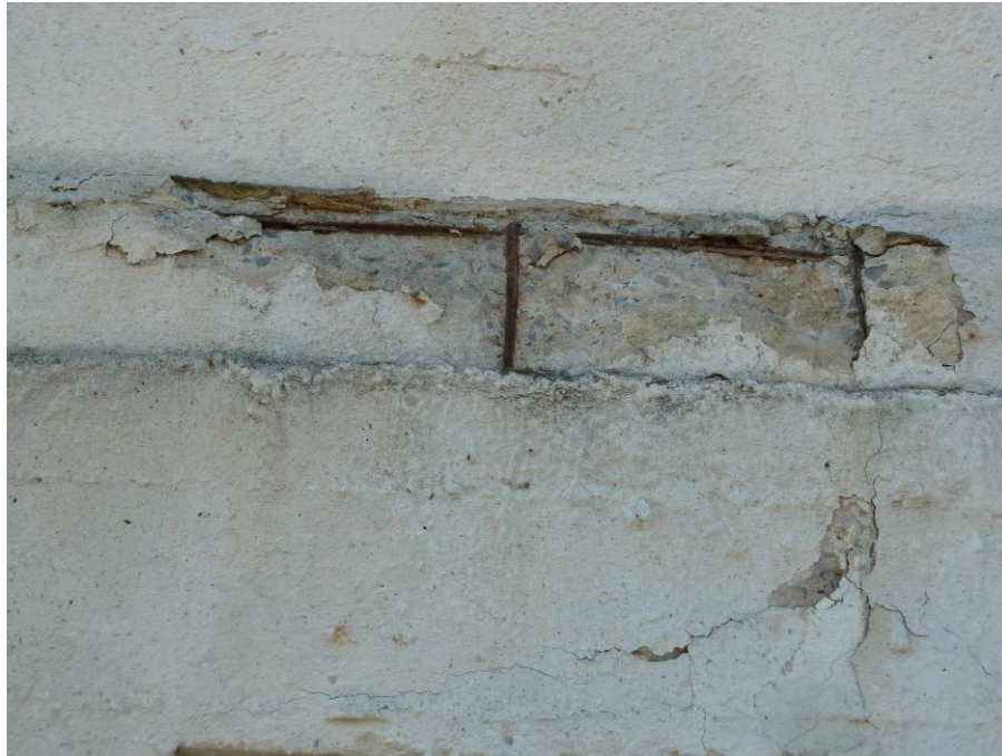
Exposed reinforcing on North Façade
