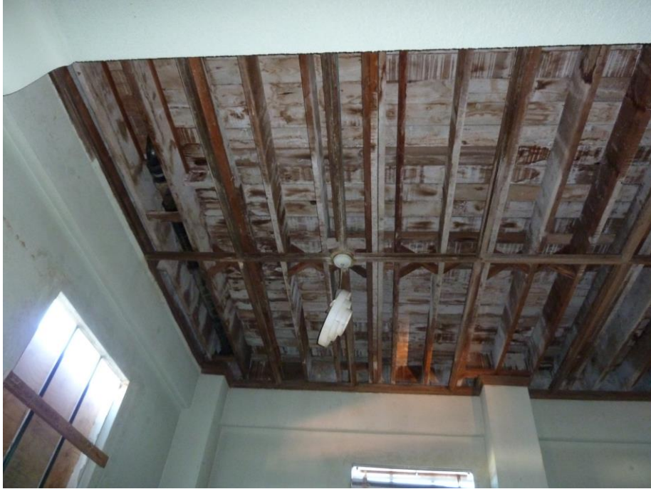
Water Damage at 2 nd Floor
