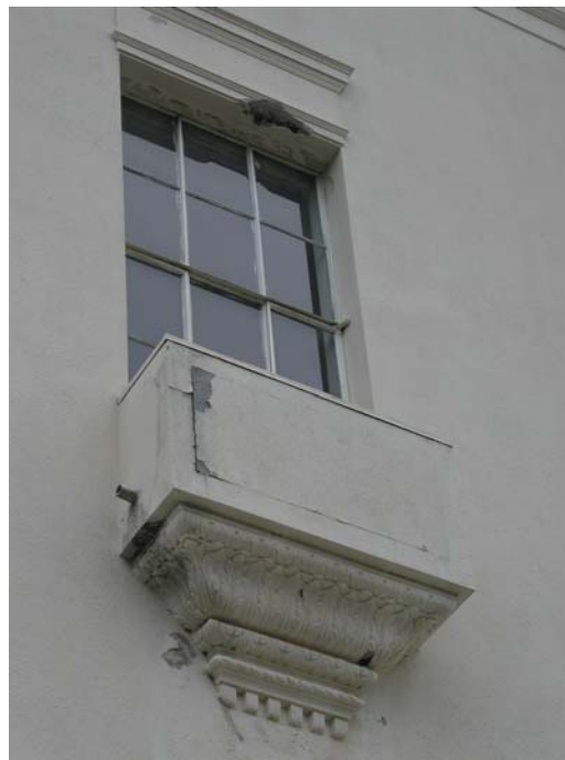
Concrete Spalling at Header (March 2008)
