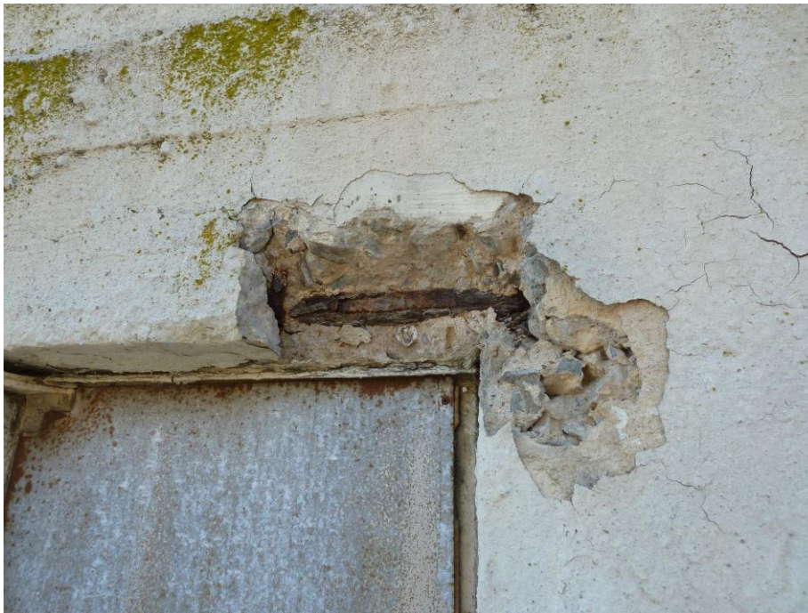
Exposed reinforcing on North Façade
