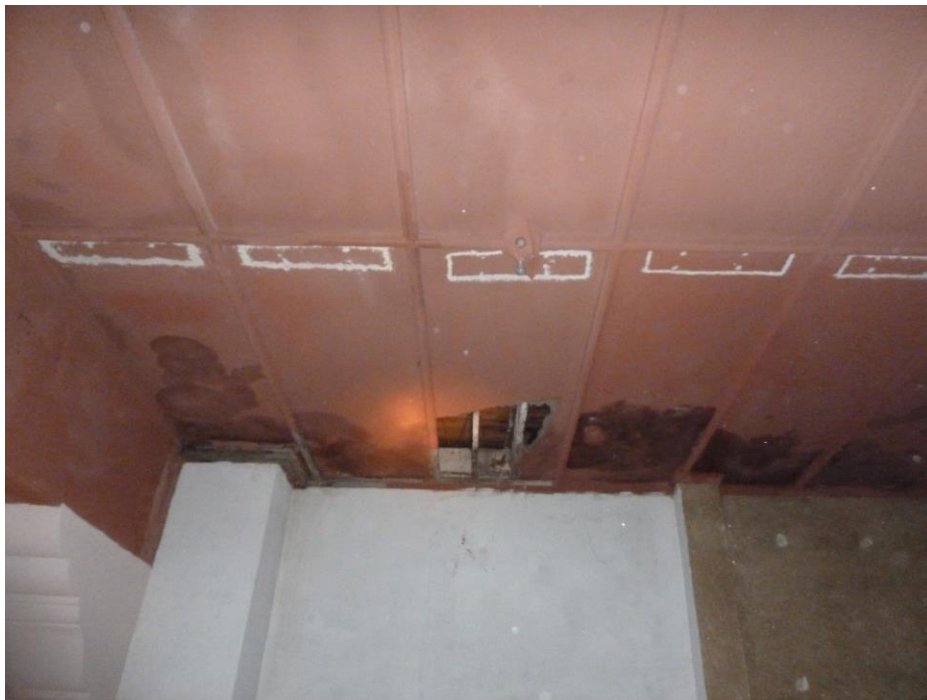
Water Damage at 2 nd Floor
