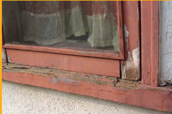
in chipping paint
