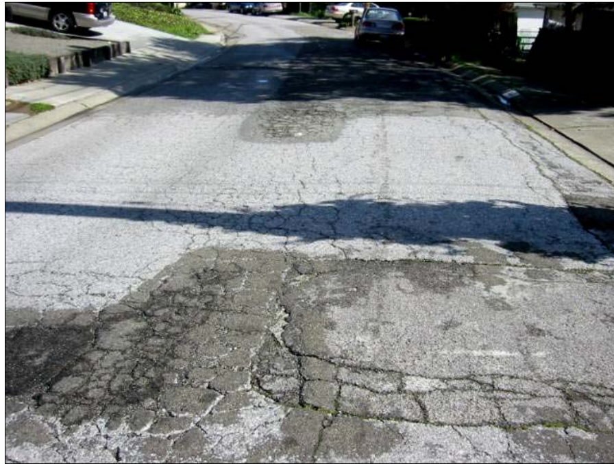
Figure 3.7 PCI <10 (Failed Condition)
