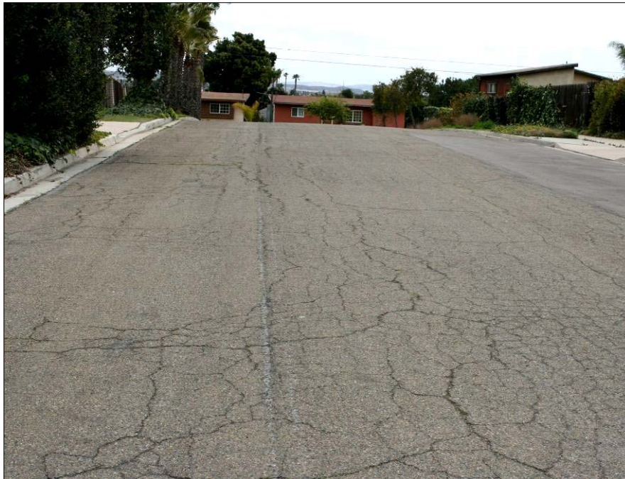
Figure 3.6 PCI = 40 (Poor Condition)
